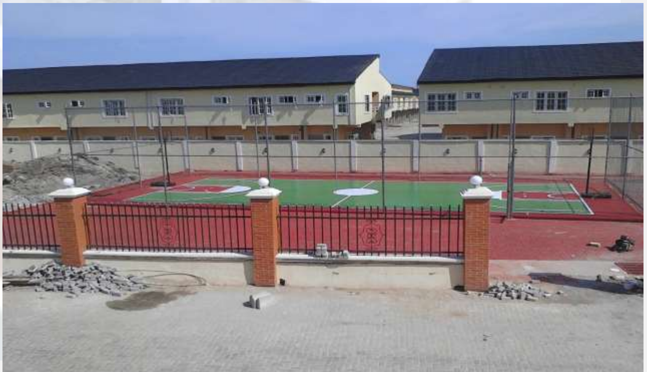
CONSTRUCTION OF RECREATIONAL FACILITIES (BASKET BALL AND LAWN TENNIS COURTS) FOR LEKKI GARDENS, AJAH, LAGOS
